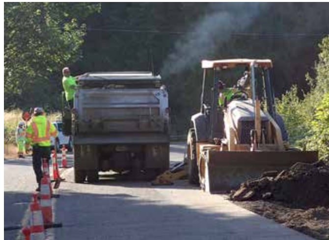
Crews worked last year to realign the curve on Cornelius Pass at NW 8th Ave. Work will resume there this year. (Photo: Mult. Co.)
