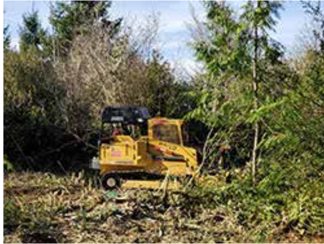
Track mulcher at work grinding old holly trees to reclaim the land on McNamee Rd. (Photo: L. Foster)
