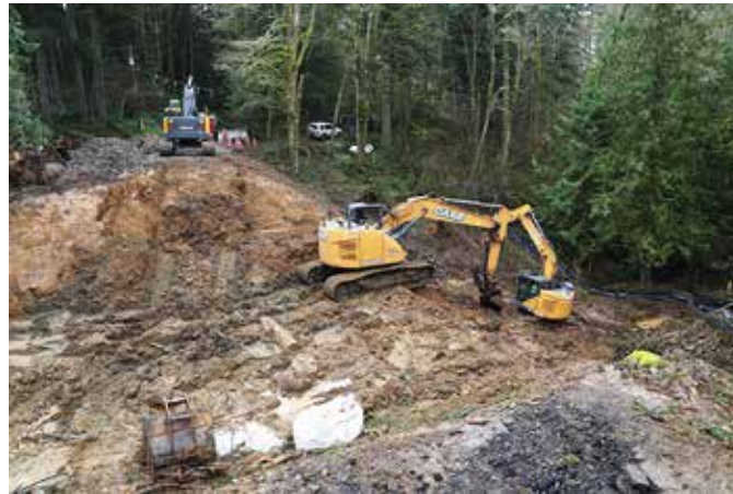
Repair of the failed culvert on upper Rock Creek Rd. required digging a VERY big hole (Photo: Mult. Co.)
